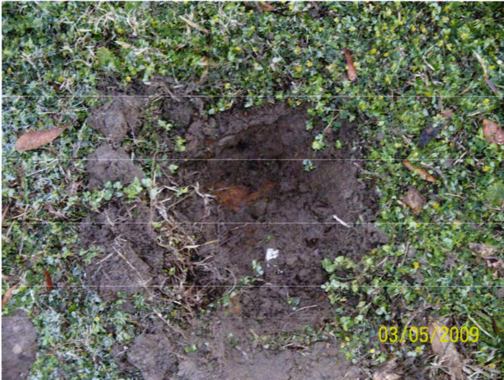
Picture 3: UST 132Banyan-2 was approximately 2 inches below ground surface.
